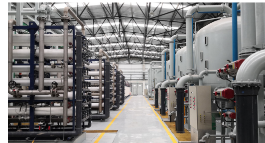
Shaanxi Longmen Coal Chemical ZLD Project
